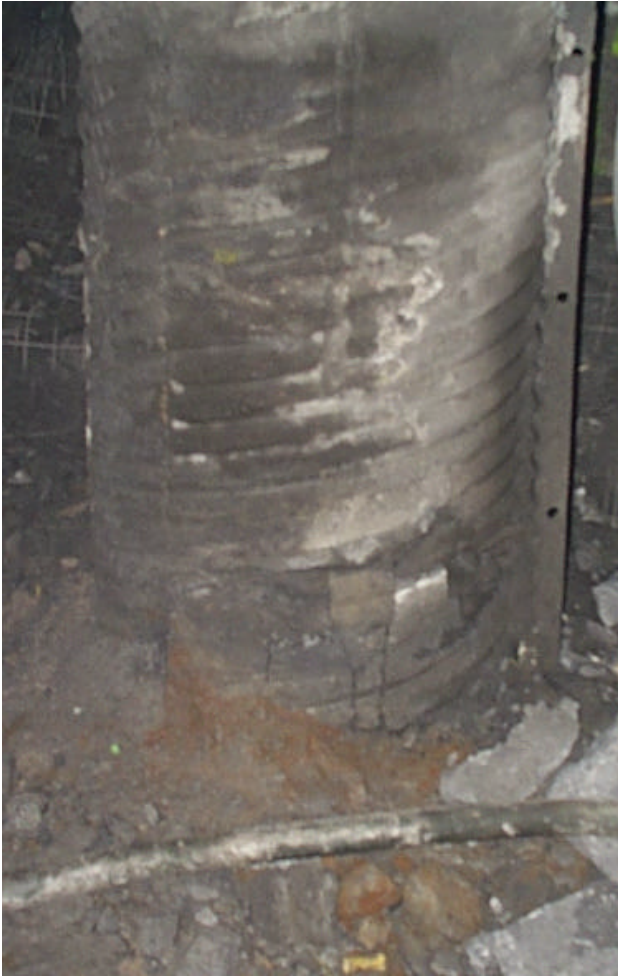
Figure 9. Crack monitoring of shotcrete pillars during mining. Failed areas marked with red paint.
