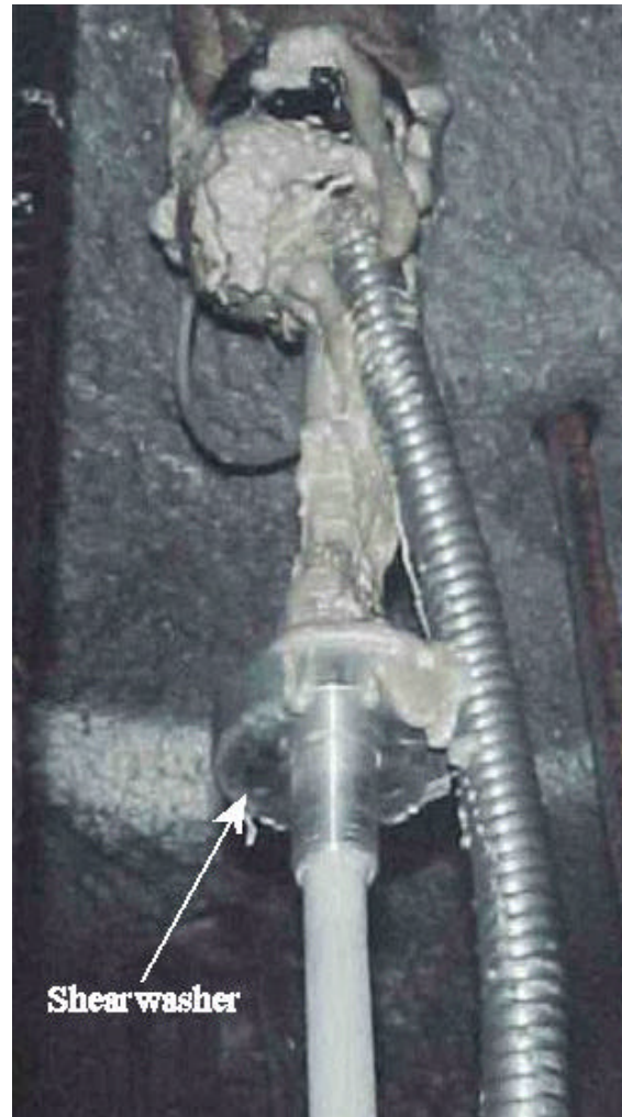
Figure 8. Closeup of Contractometer installation in stope back showing foam used to fix instrument head and last anchor in the hole. Note the use of shear washers on the anchors within the shotcreted portion of the pillar.
